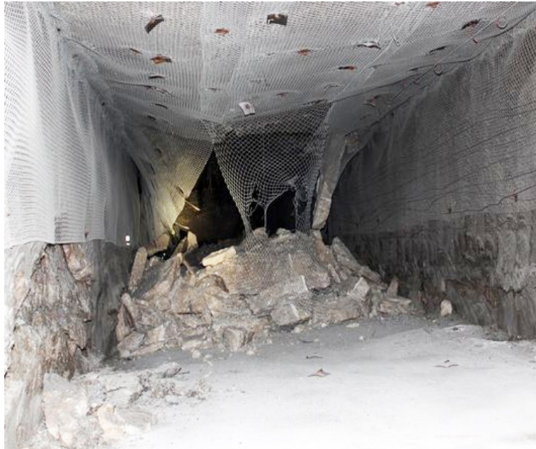
One of two deep-underground tunnel roof collapses that recently caused evacuations of the military radioactive “Waste Isolation Pilot Plant” in New Mexico. Photo: Energy Dept.
